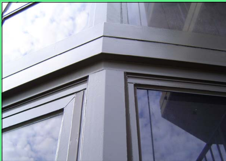
Pre-cured room-temperature vulcanized (RTV) silicone sealants have been used to repair severe water-intrusion problems in aluminum window systems with numerous metal-to-metal joints. With the correct finish specification, the sealant should not be noticeable.
